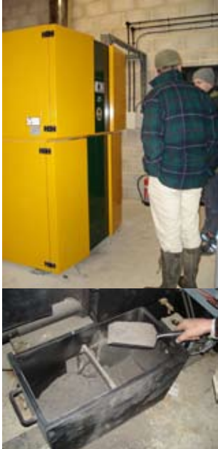
Top down: Robin Thorpe, whilst researching for a replacement for the oil-fired boiler at 7 Sisters Country Park, was delighted to see John Leigh-Pemberton's recently installed 150kw automated wood fired boiler in action; occasional removal of ash, only 4 bags a year, a useful bi-product for the garden.
